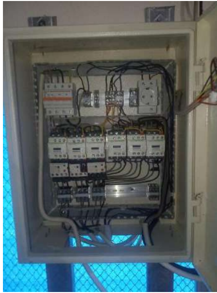
Figure 3. Contactor panel unit.
