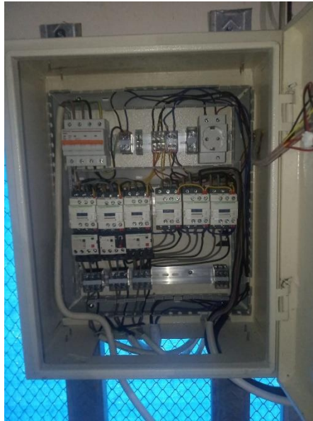
Figure 3. Contactor panel unit.
