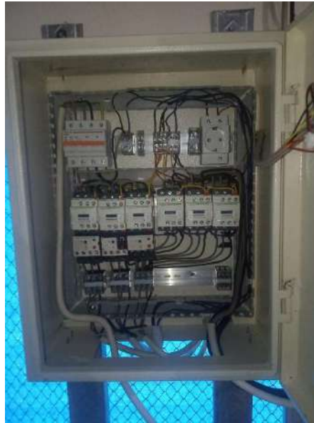
Figure 3. Contactor panel unit.
